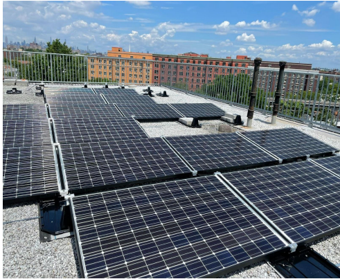
Community Solar System
